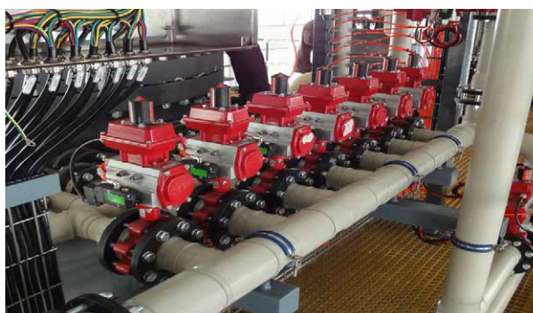
Filtrate outlets including sight glass for each outlet. Outlets are grouped into headers with individual pneumatically actuated valves leading into the filtrate collector.
