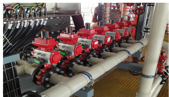
Fig. 3: Filtrate outlets including sight glass for each outlet. Outlets are grouped into headers with individual pneumatically actuated valves leading into the filtrate collector.
