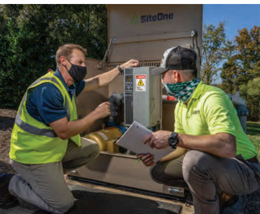
Rinschler spends the majority of his time working on projects involving pump systems, rainwater harvesting, retrofits and more advanced irrigation control systems.
