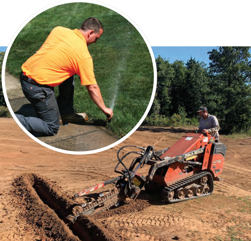
Before beginning any trenching work, make certain to locate all underground utilities such as cable, electricity, gas, water and sewer. Give utility companies plenty of time to respond. Photo, top: Aqua-Lawn Inc., below: Poseidon Irrigation Oklahoma
